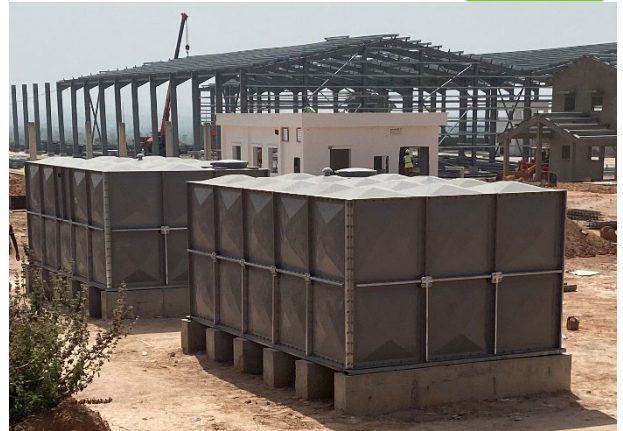
OCP Africa's fertilizer blending plant facility under construction in Kaduna State. Photo credit: OCP Africa
