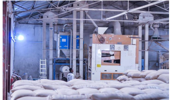
Adefunke Desh will leverage part of the Trade Hub's co-investment to upgrade its grain cleaning equipment in Kaduna State.
