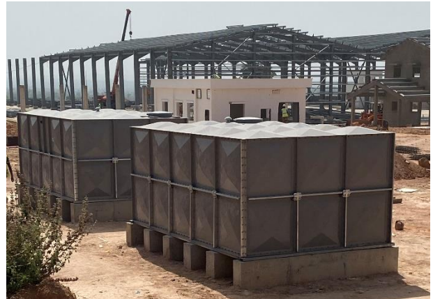
OCP Africa fertilizer blending plant facility under construction in Kaduna State. Photo credit: OCP Africa
